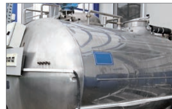
z.B. TANKANLAGE e.g. STORAGE TANKS
